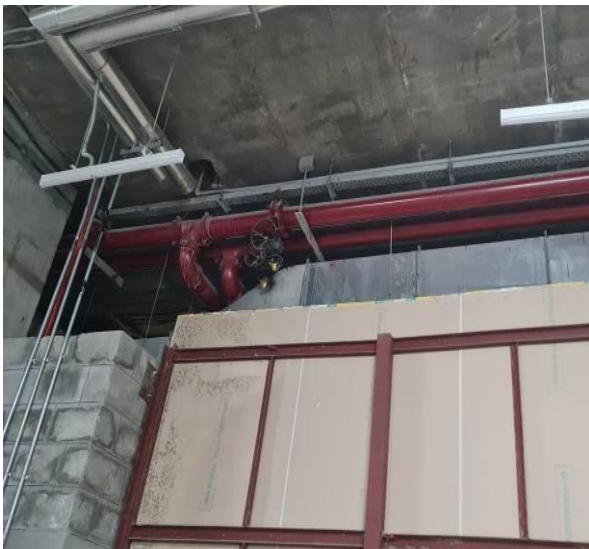
Space equipped with Fire Fighting Lines / FHC
