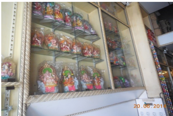
Photo 5 Covered with Materials, Wall No. 1 of Shop No. 92A, Ground Floor
