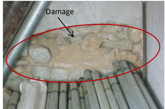
Photo 2 Damage of Wall No. 4 of Shop No. E62, Ground Floor
